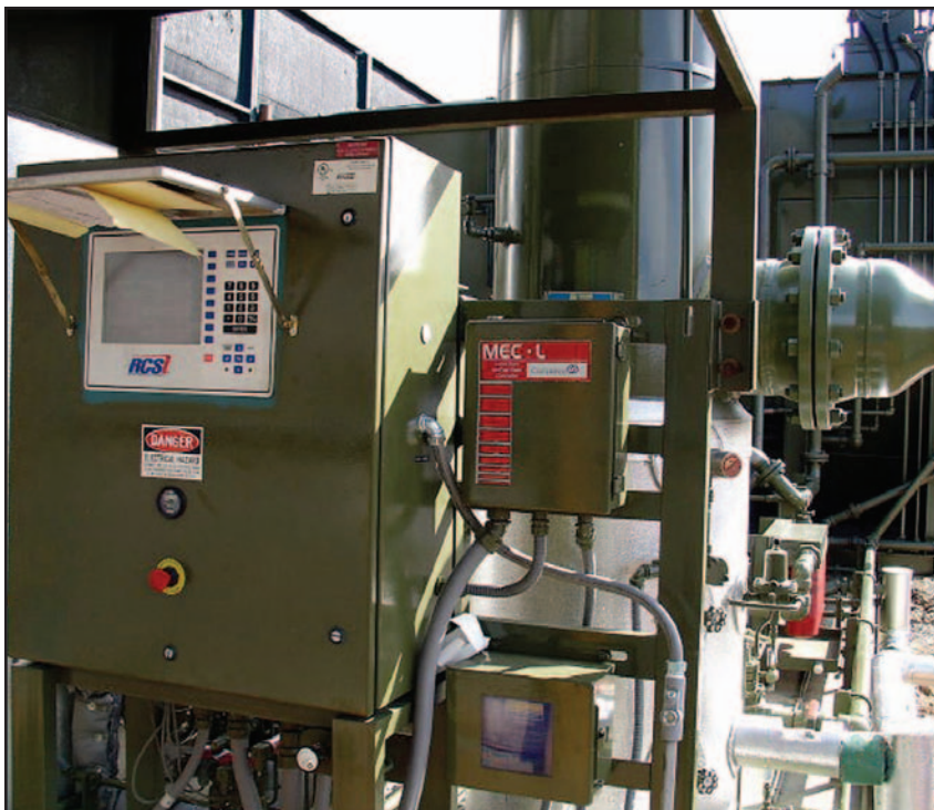
■ The Compliance Controls MEC-L Air Fuel Control System control box, installed at a coal-seam methane compression facility in the San Juan Basin of the four-corners area.
